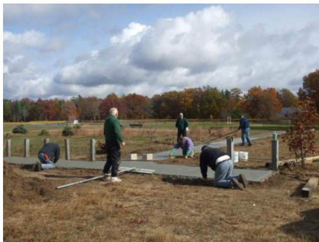
Members putting in walkways at Mullally Park in Laketon Township. Lions Ron Hansen, Dennis Cobler, Dennis Loughridge, Larry Seastrom, Denny Bates and Ed Mouw
